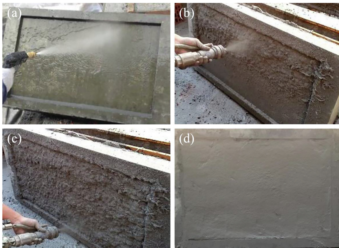
Fig. 3. Spray process of the UHTCC: (a) the surface of the existing concrete is cleaned using a water jet; (b) UHTCC is sprayed; (c) spraying is completed; (d) the surface is smoothed.
