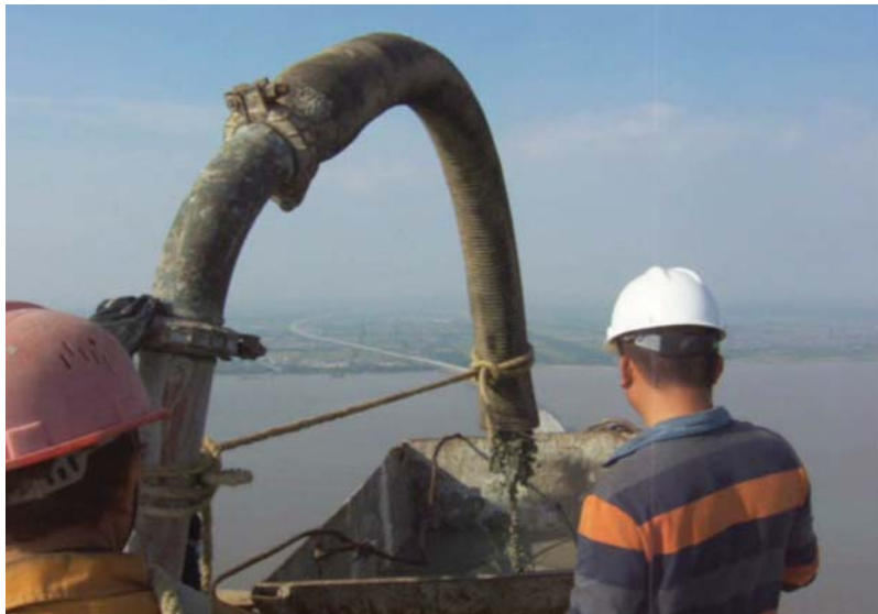
Figure 3-29 Pumping of fiber reinforced concrete to a height of 306m at Su-Tong Bridge, Suzhou, China (Photo provided by Jinyang Jiang)
