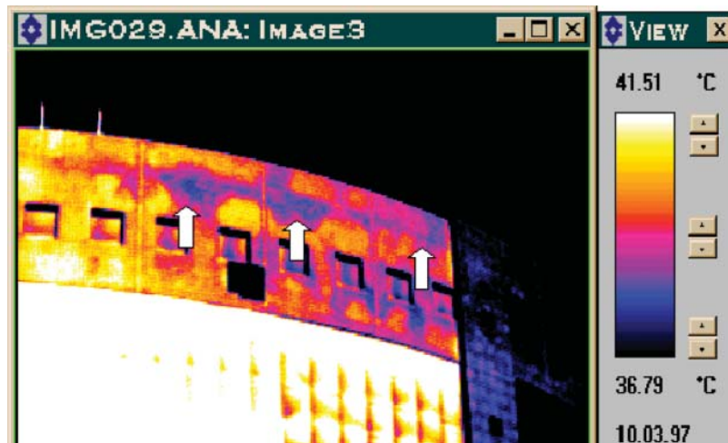
Figure 8-49 The lower-temperature areas (indexed by upward arrows) indicating the defect areas filled with water or moisture
