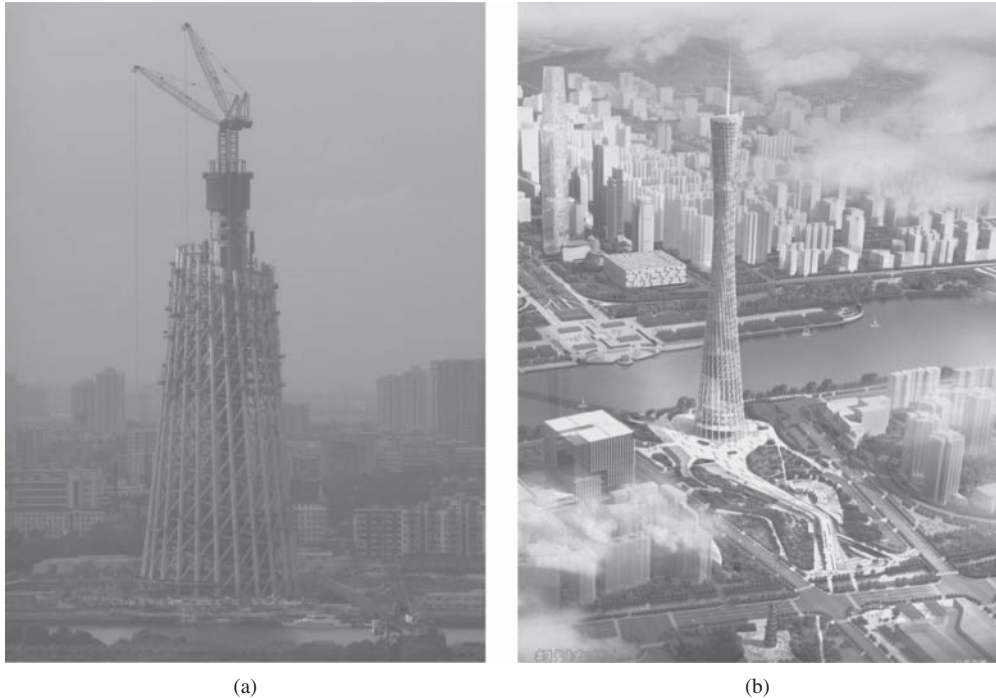
Figure 6-54 Guangzhou TV Astronomical and Sightseeing Tower: (a) under construction; and (b) site view of finished tower (Photo provided by Linhai Han)
