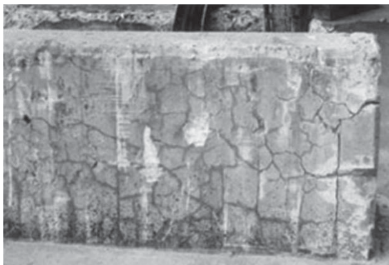
Figure 5-72 Cracks caused by AAR. (Source: Thomas and Folliard, 2007, 247-281 / with permission of ELSEVIER.)
