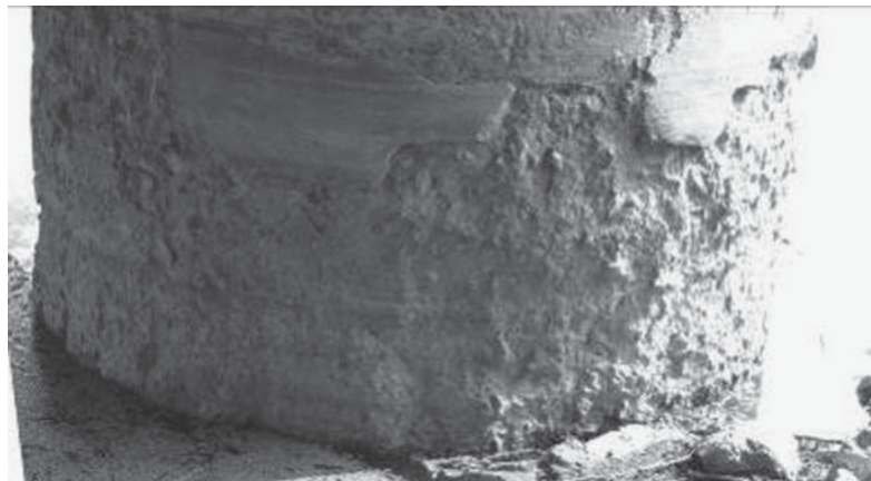
Figure 5-74 Scaling deterioration caused by freezing-thawing
