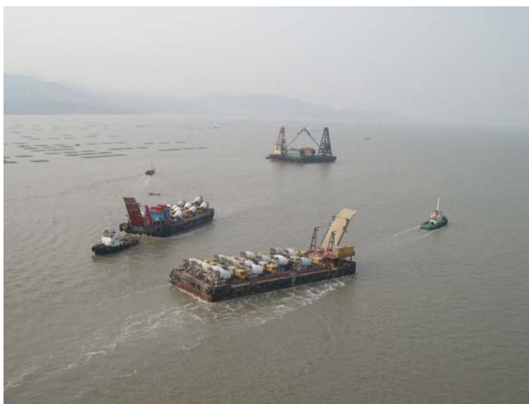
Figure 3-23 Delivery of concrete to an ocean construction site using a ferry (Photo provided by Ove Arup, HK)
