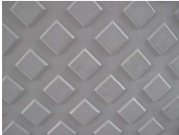
Figure 6-33 Application of UHSC in pavement cover plate in high-speed railway in China
