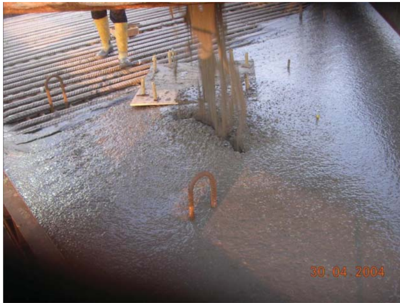
Figure 6-42 Application of self-compacting concrete for in situ construction of a pile cap (Photo provided by Ove Arup, HK)
