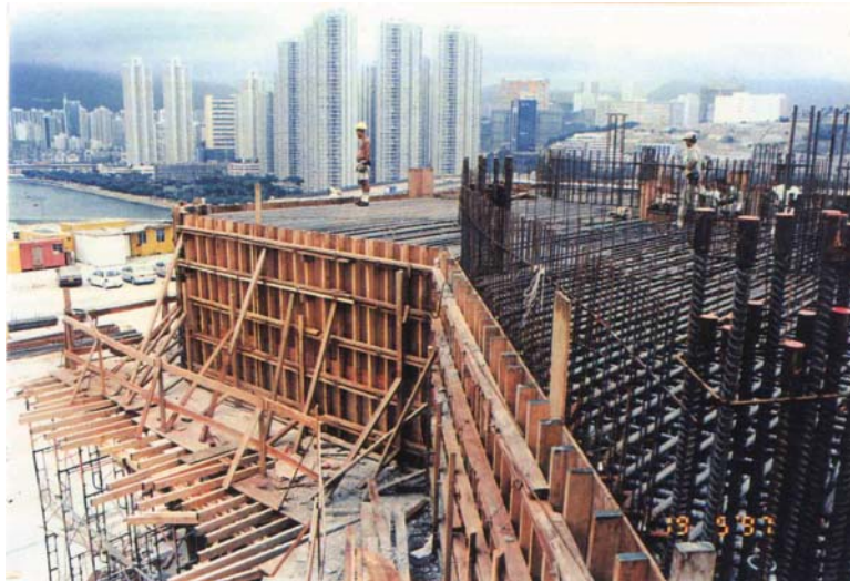
Figure 3-24 Formwork for transfer block of a tall building (Photo provided by Mr. Peter Allen)
